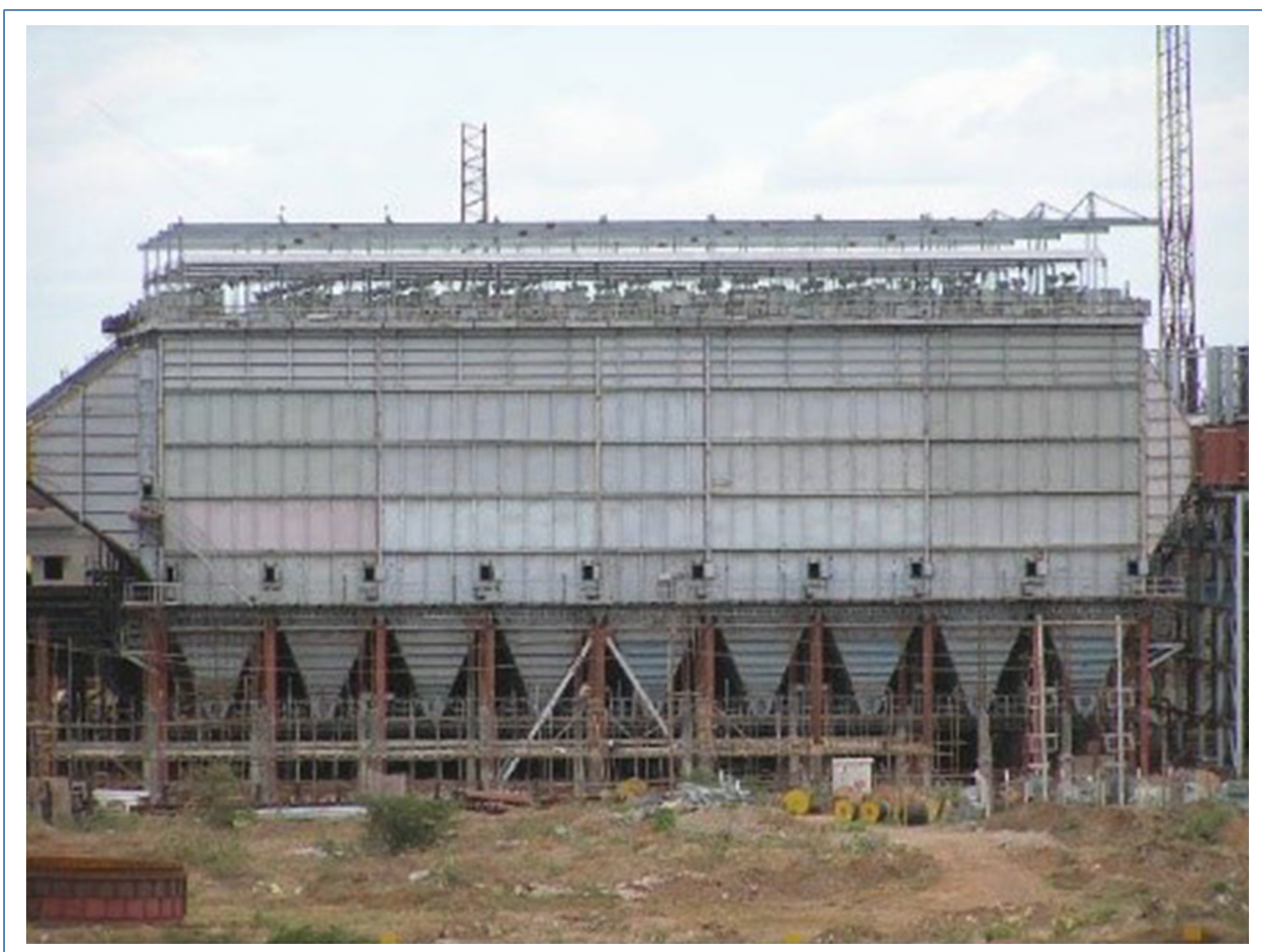
Figure E5. High-efficiency Electrostatic Precipitator (ESP) installed by BHEL in a TPP in India
