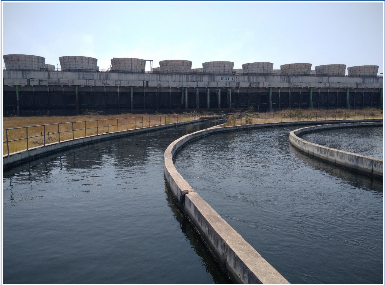
Figure 4: Circulating Water Forebay and Induced Draft Cooling Towers in Yeramarus TPS
