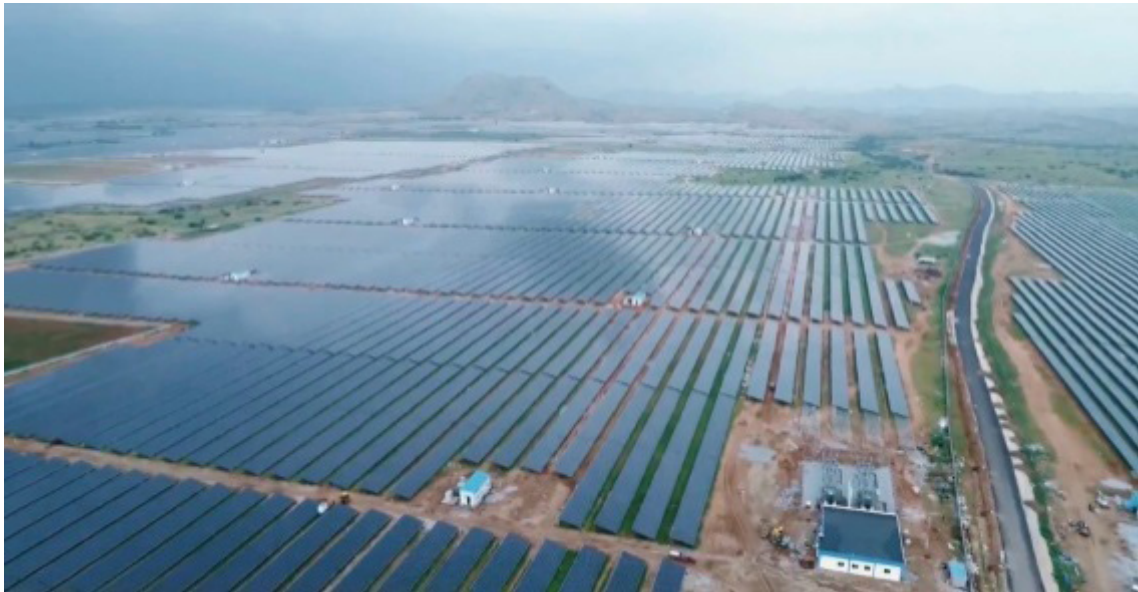
The Largest Solar Power Plant in India in Pavagada, Karnataka.
