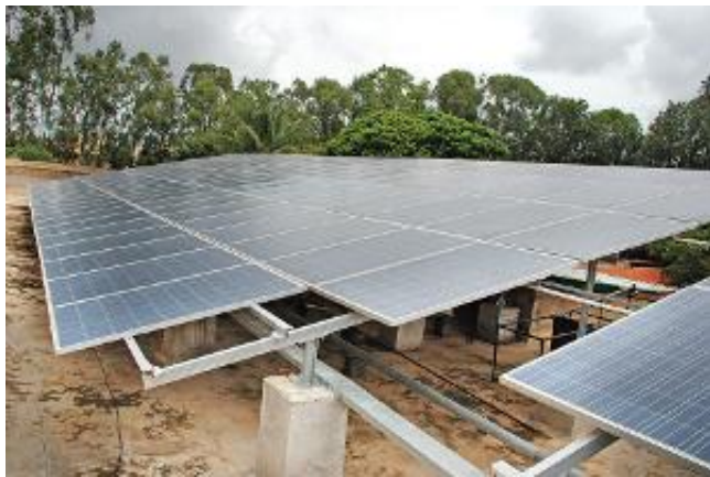
Grid tied solar rooftop plant (NIAS guesthouse block)
